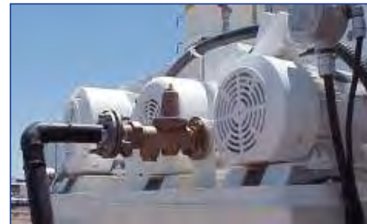
NOx Water Supply (2" pipe)
